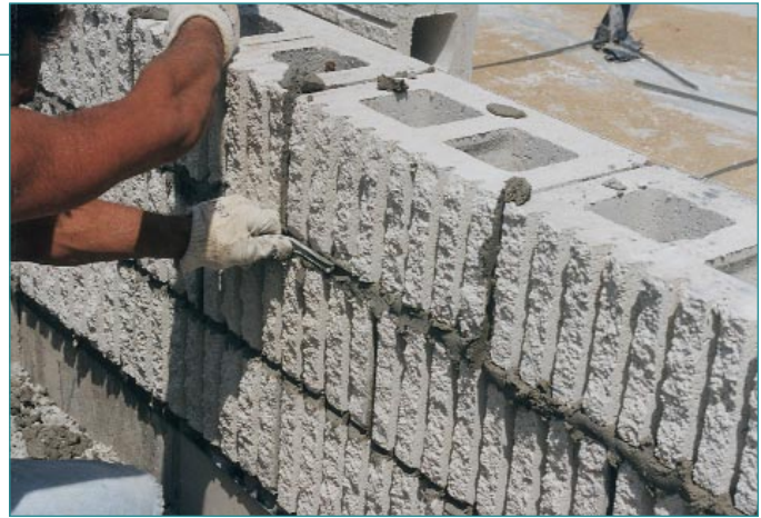
Figure 2. Tooling joints compacts the mortar and creates a weather-tight bond. This minimizes water entry into the wall, which reduces the potential for efflorescence. (IMG14594)
