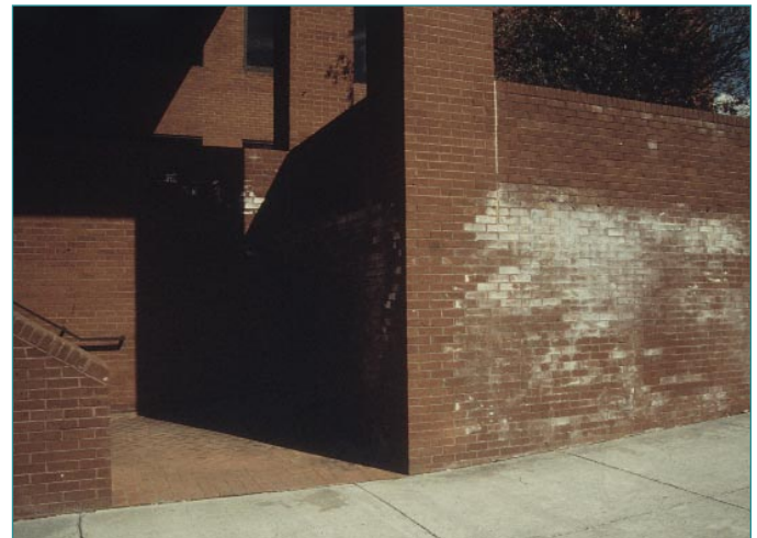
Figure 1. Efflorescence is often called “new building bloom” because it appears on fresh masonry surfaces. (IMG14593)
